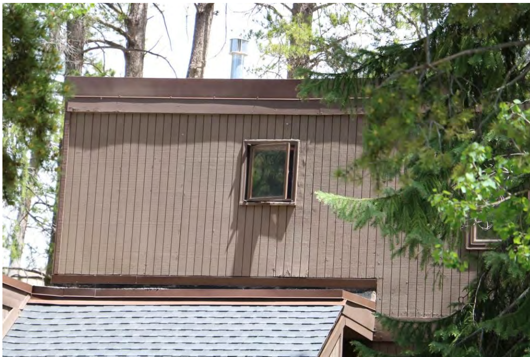
Upper portion of front (west) elevation, illustrating exterior wall cladding and casement windows, view facing east.
