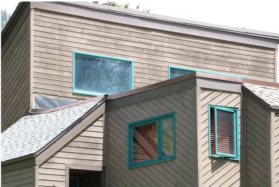
Detail illustrating the horizontal and diagonal wood cladding as well as the range of window types, including wood-frame fixed and casement examples, view facing northeast.
