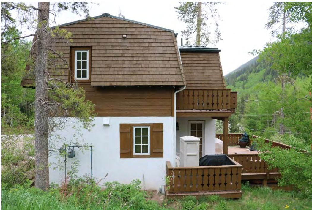
Side (northwest) and rear (southwest) elevations showing the recently added wood decks, view facing southeast.
